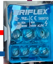
Bus / Termination Point
